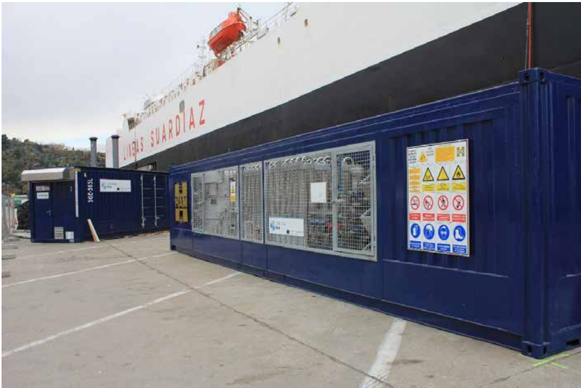
Figura 158. Pilot of 1 December. Equipment.
