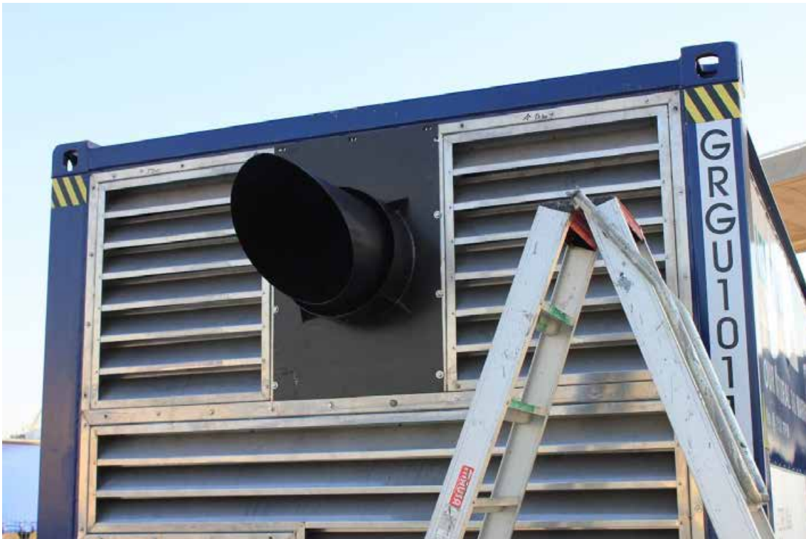
Figura 135. Installing the exhaust gas pipe. The grilles are part of the engine room ventilation system.
