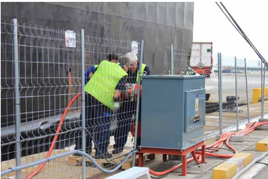
Figura 159. Pilot of 1 December. Connection of the medium voltage cable from the ship to the connection terminal.
