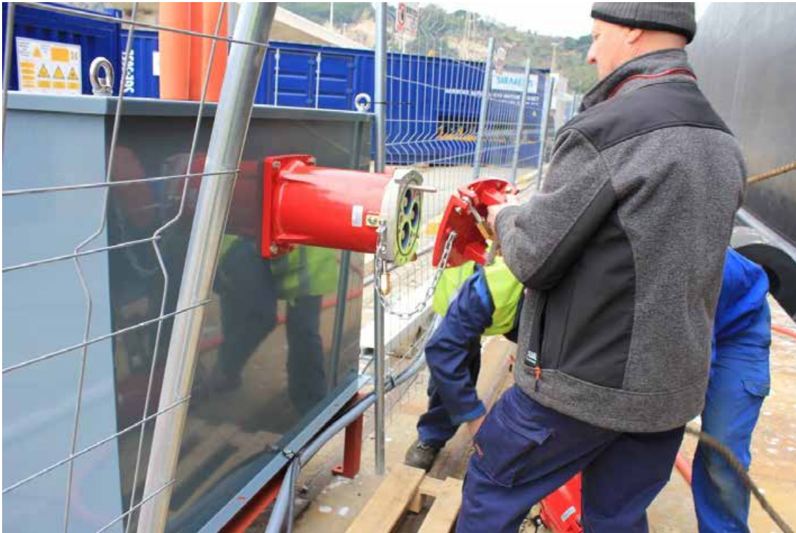
Figura 97. Disconnection between the connection terminal and the cable coming from the ship. Connector protection.
