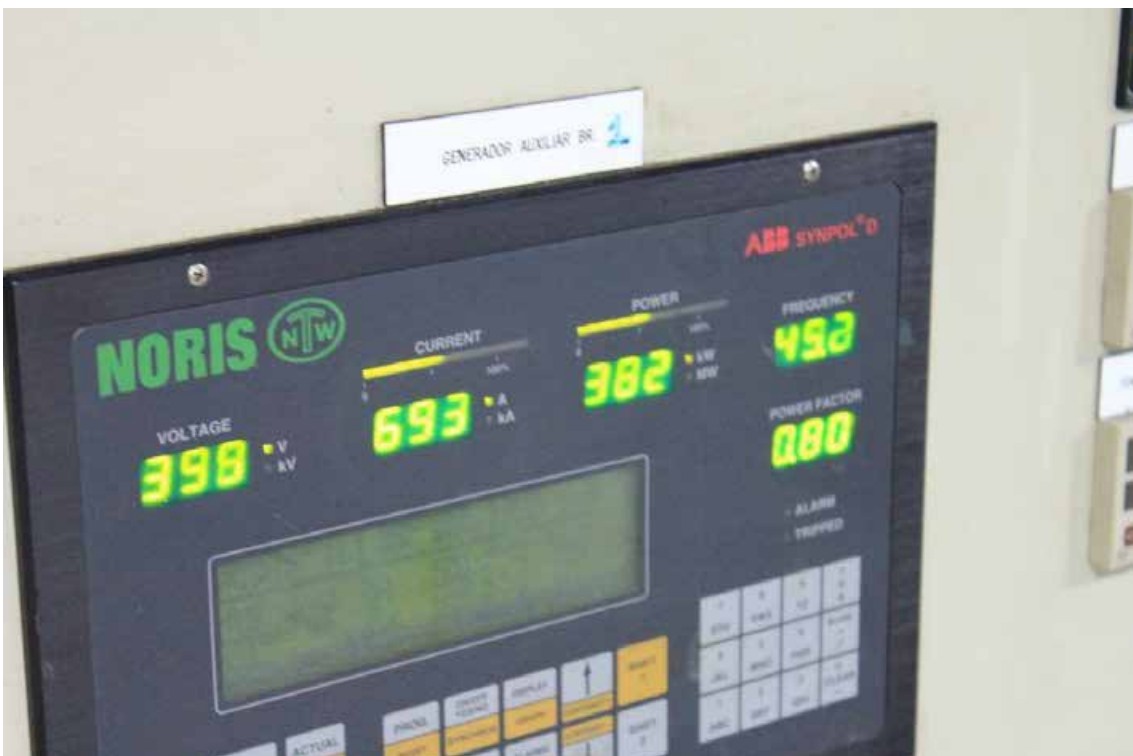
Figura 167. Pilot of 8 December. Control panel on board the gas engine. Power 382 kW, 398v and frequency of 49.2 Hz.
