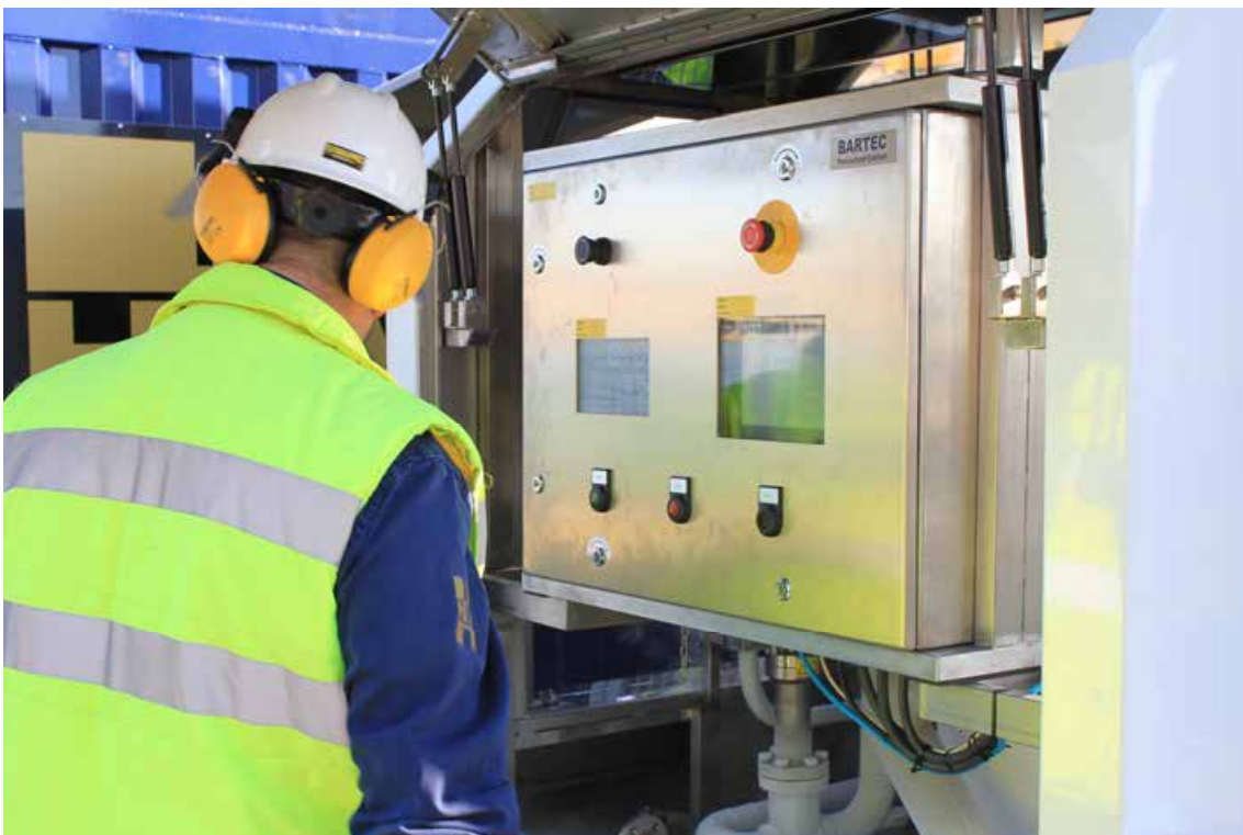
Figure 18. Mobile service station. Detail of the dispenser and control panels.
