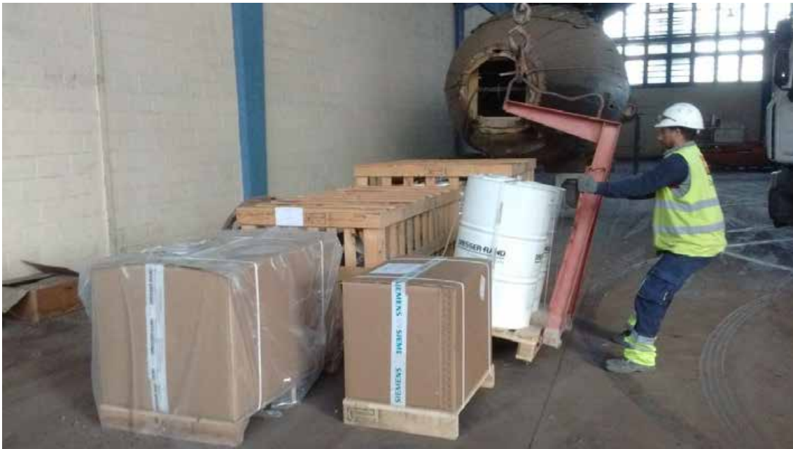
Figura 24. Storing Guascor-Siemens equipment and materials on Sant Bertran.
