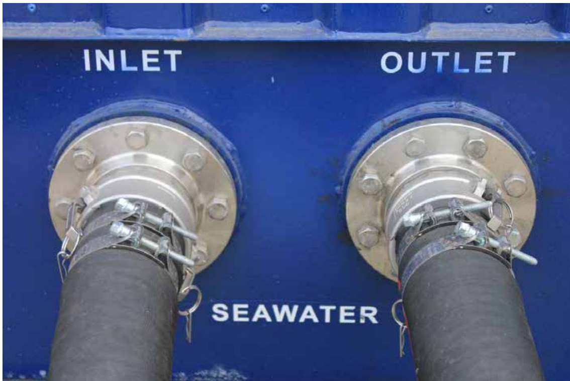
Figura 63. Installing the ND100 pipes of the secondary refrigeration circuit. Connection to entry and exit point using flanges.
