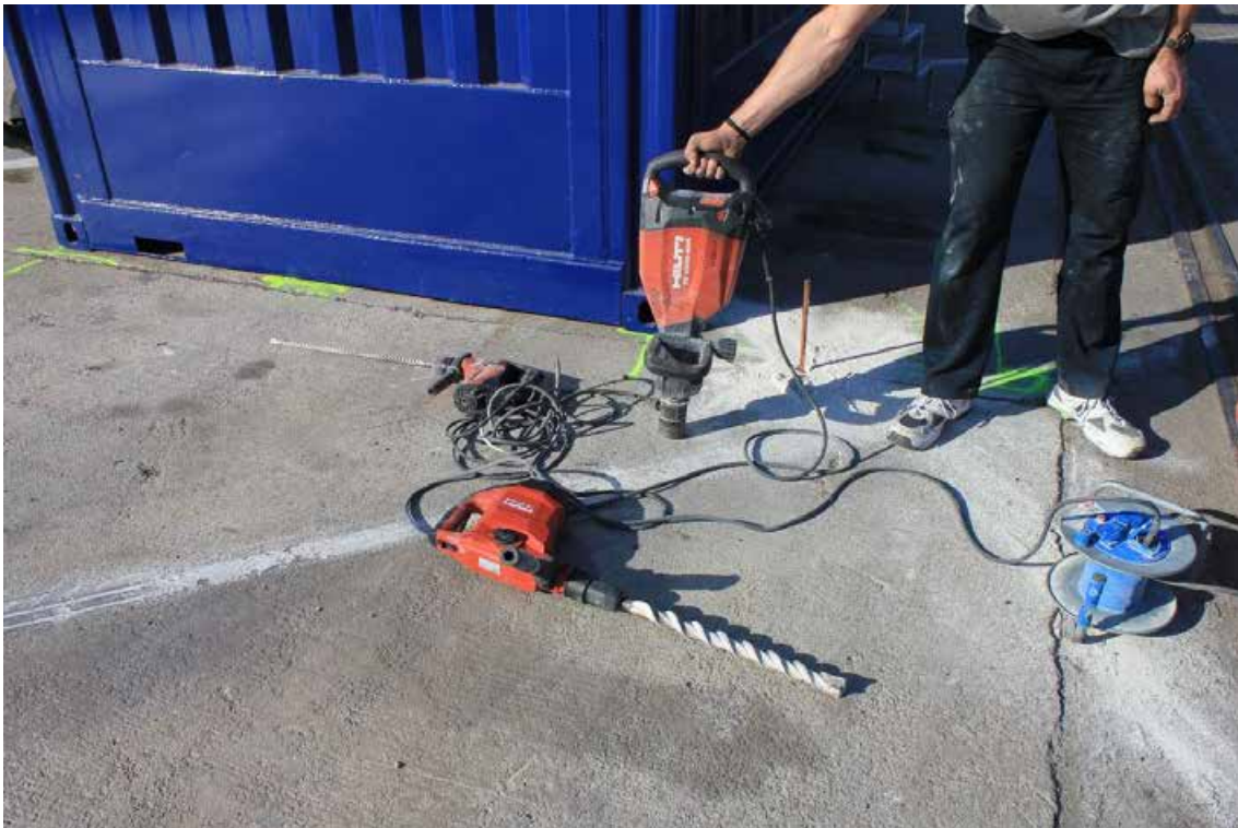
Figura 55. Drilling in the concrete slab of the wharf to drive the copper earthing rod.
