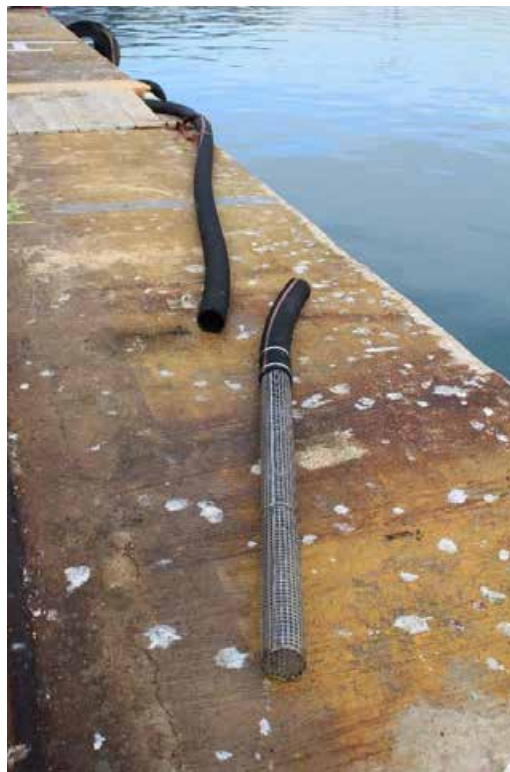
Figura 64. Detail of the particulate filter at the end of the inlet pipe.
