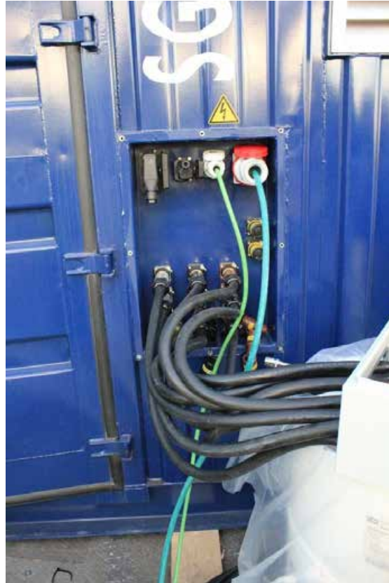
Figura 140. Connection of the 400v output cables to the junction box.
