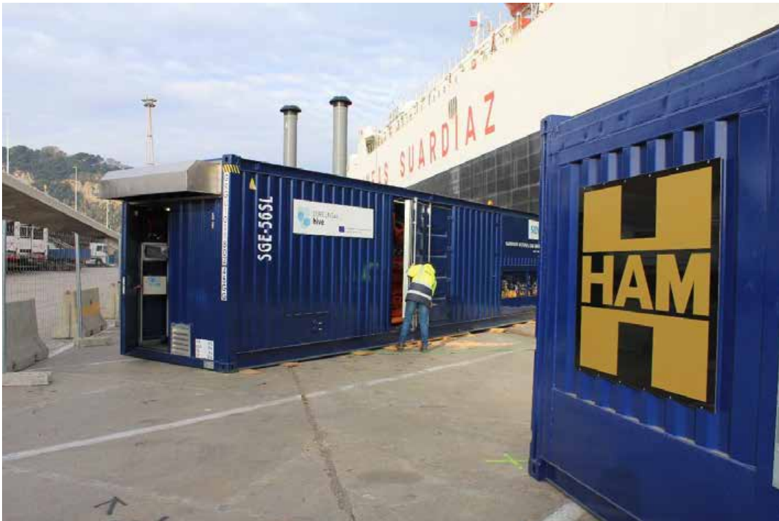
Figura 172. Pilot of 15 December. Starting the generator engine.
