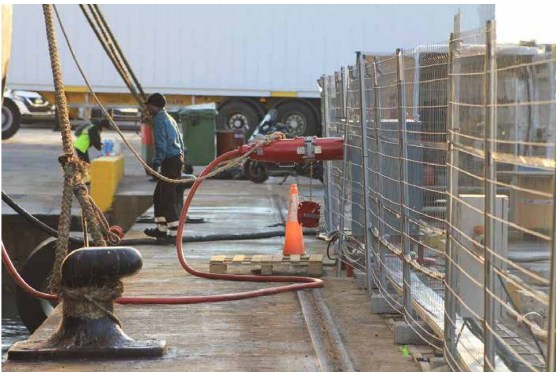
Figura 171. Pilot of 15 December. Connecting the medium voltage line to the connection terminal.
