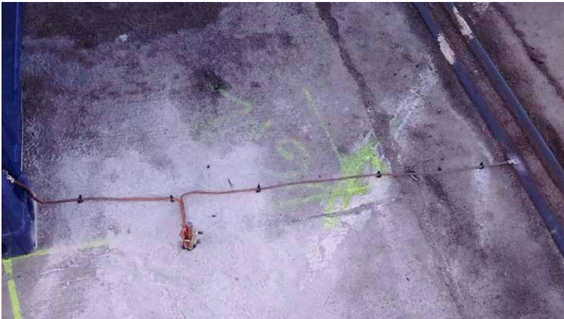
Figura 56. Gas container earth. Union of the copper rod with the train tracks and with the tank container earth connection.
