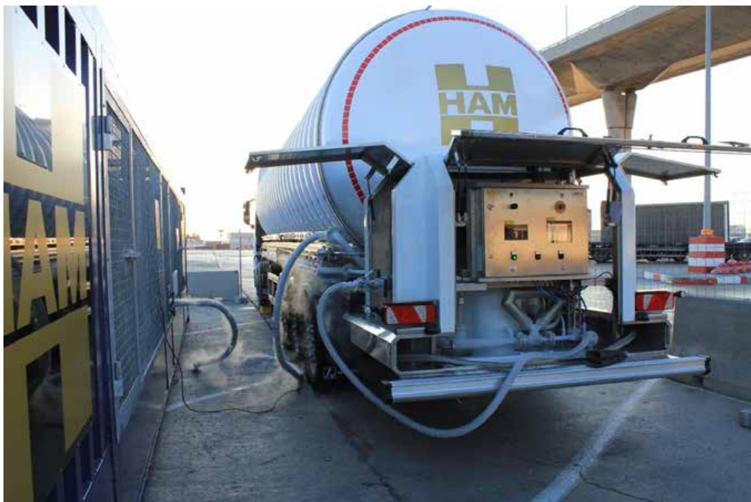
Figura 122. Tank control system. Pipes cooled by the passage of LNG to -145^{\circ}\text{C} .
