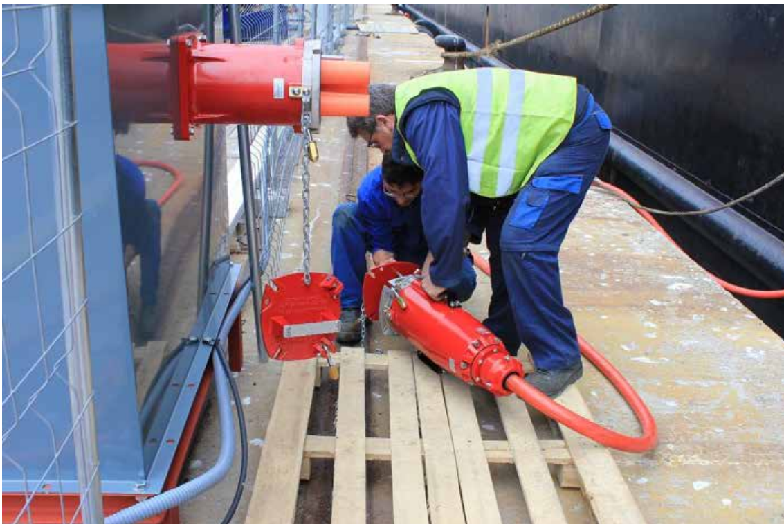
Figura 96. Disconnection between the connection terminal and the cable coming from the ship. Connector protection.
