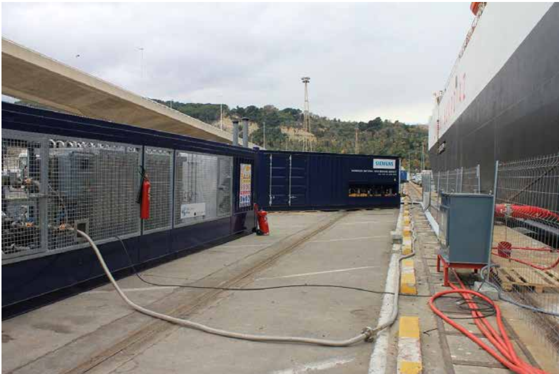
Figura 77. Gas hose between the tank container and the engine container.
