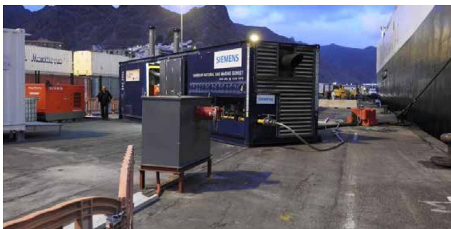
Figure 60. Pilot of the 11th of November. Set of equipment.
