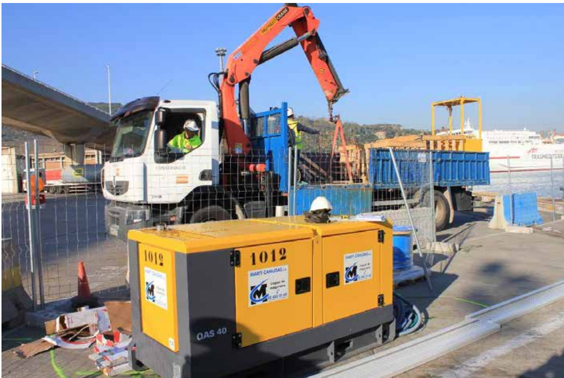
Figura 44. Rental generator Europa-Atlas-Copco QAS40 generators.
