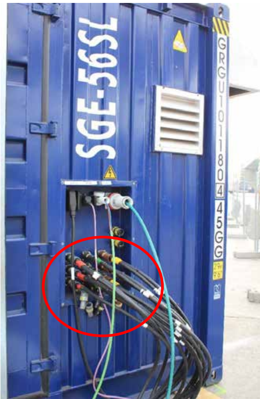
Figura 81. 400 Vac generator engine voltage output connections (3 phases, positive, negative and neutral).
