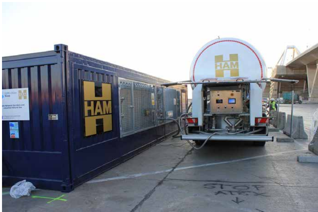
Figura 120. Ground clamp connection and connection of the LNG hose to the container inlet valve.
