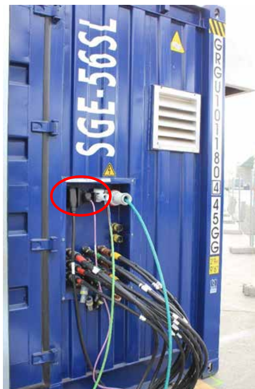
Figure 46. Control signal between the engine container and the ship (through the transformer).
