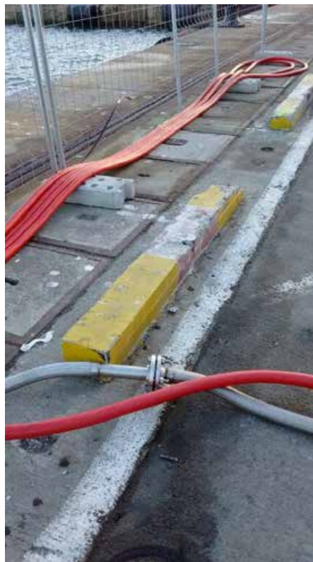
Figura 90. 15 kV wiring between earth transformer and connection terminal.
