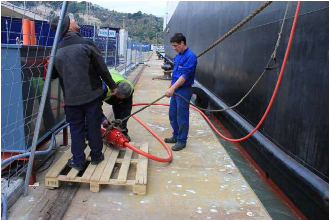
Figura 160. Pilot of 1 December. Disconnection of the medium voltage cable.
