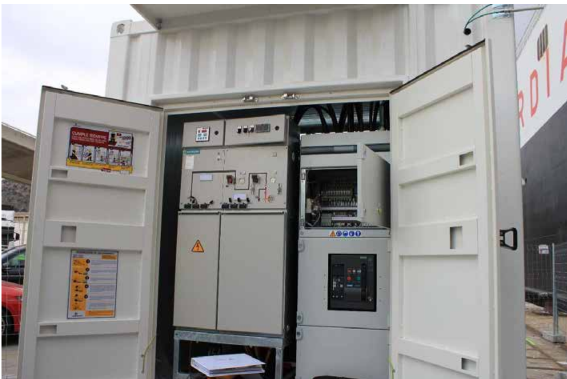
Figura 86. Earth transformer. Control panels.
