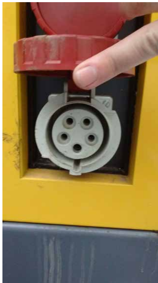
Figura 46. 400v generator connector.
