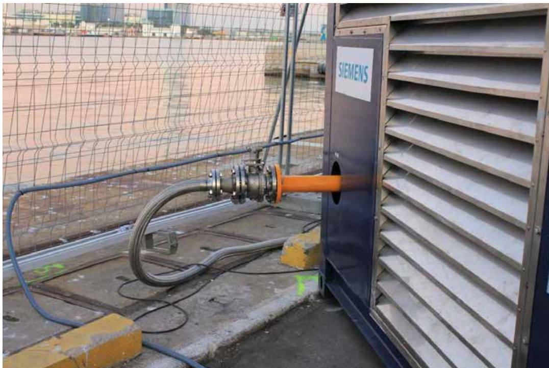
Figura 74. Gas inlet to the gas train of the engine container. Manual shut-off valve and reducer.
