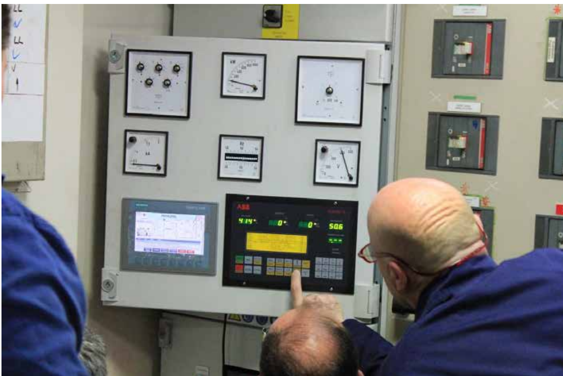
Figura 165. Pilot of 8 December. Control panel on board the auxiliary gas engine.
