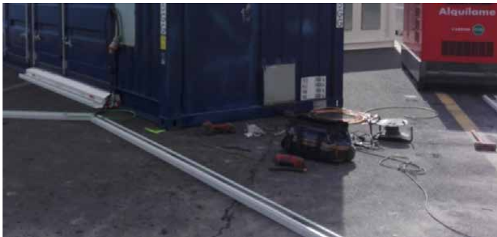
Figure 6. Engine container placement signage (Siemens).
