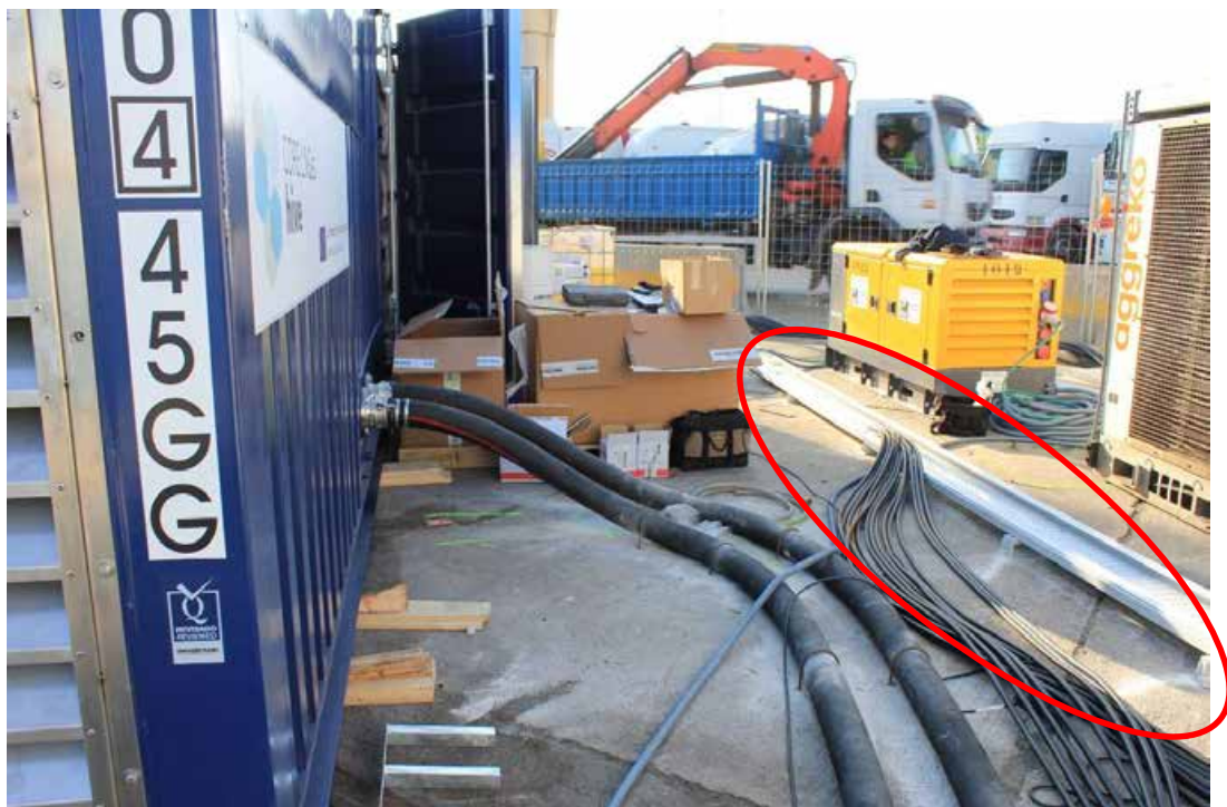
Figura 82. Surface channelling of the wiring between the generator engine and the earth transformer.
