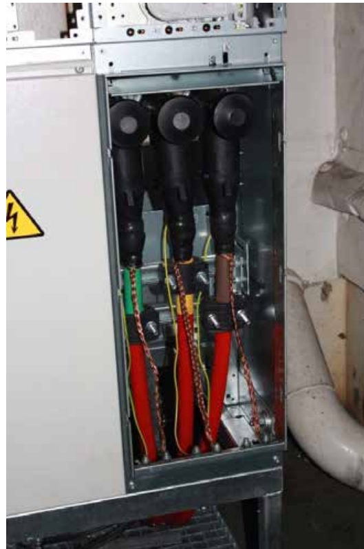
Figura 101. Ship's transformer. Detail of the connection point of the 15 kV cable from the connection terminal.
