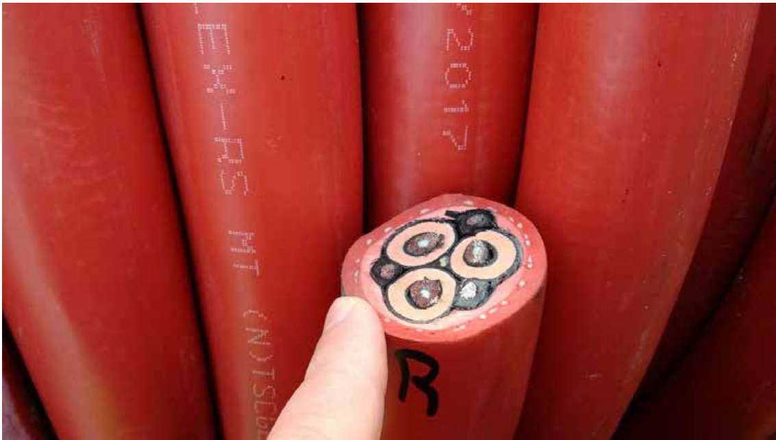
Figura 91. 15 kV wiring between earth transformer and connection terminal. Detail of the copper radial field conductor 3 \times 25 + 3 \times 25 / 3 \text{mm}^2 .
