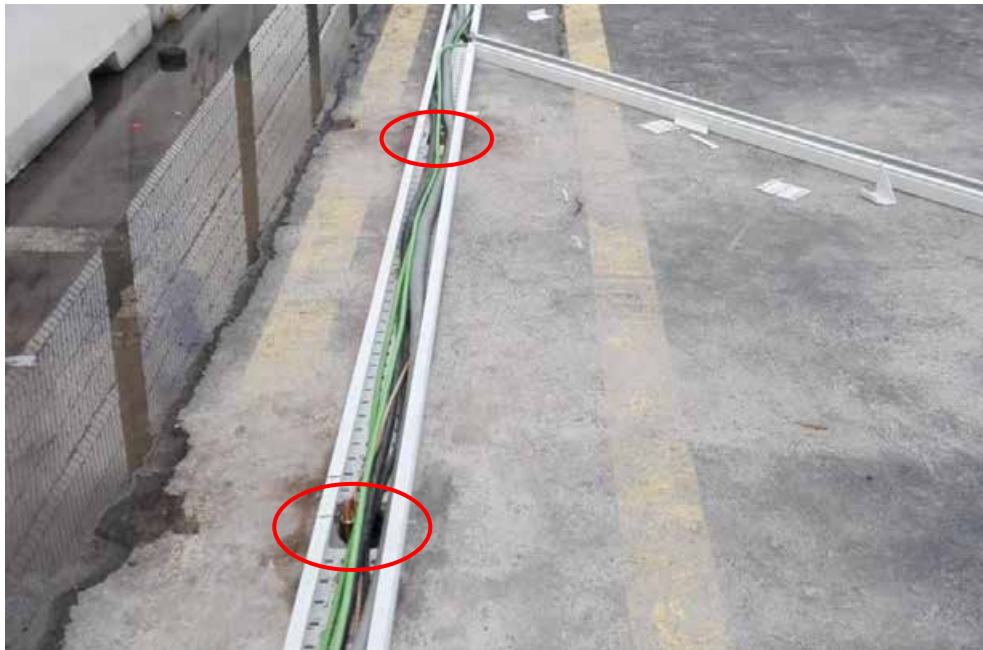
Figure 29. Gas container grounding. Connection the electrode with the ground system of tank container.
