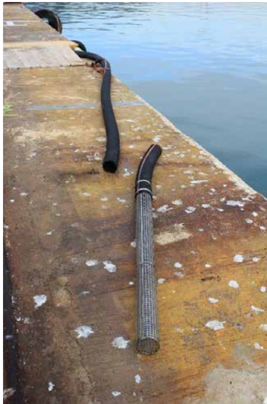
Figure 32. Detail of the particulate filter at the end of the inlet pipe.
