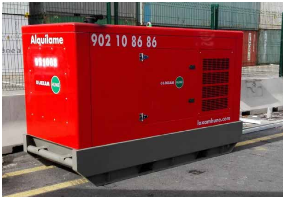
Figure 20. Loxam Hune rental generator
