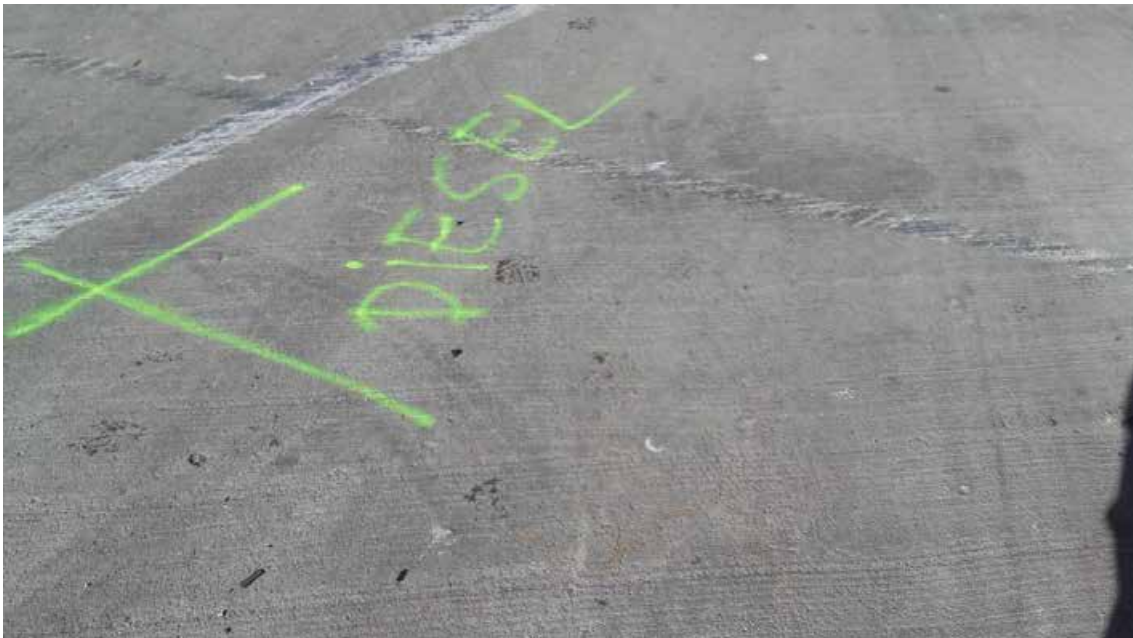
Figura 12. Marking the position of the diesel generator to supply electricity to the ensemble.
