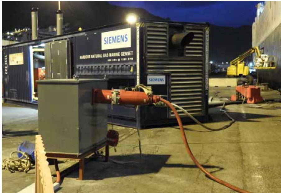
Figure 63. Pilot of the 11th of November. Connection of the medium voltage cable to Monaguillo .
