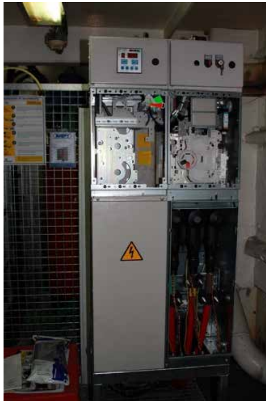
Figura 100. Ship's transformer (installed).
