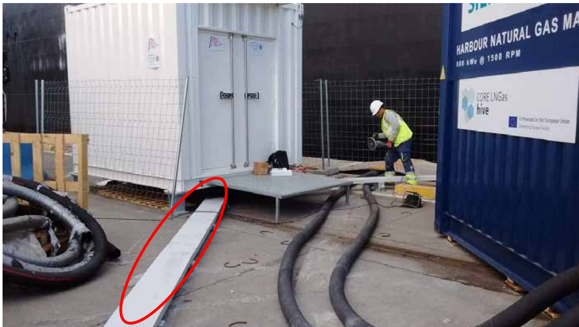
Figura 84. Surface channelling of the wiring between the generator engine and the earth transformer.
