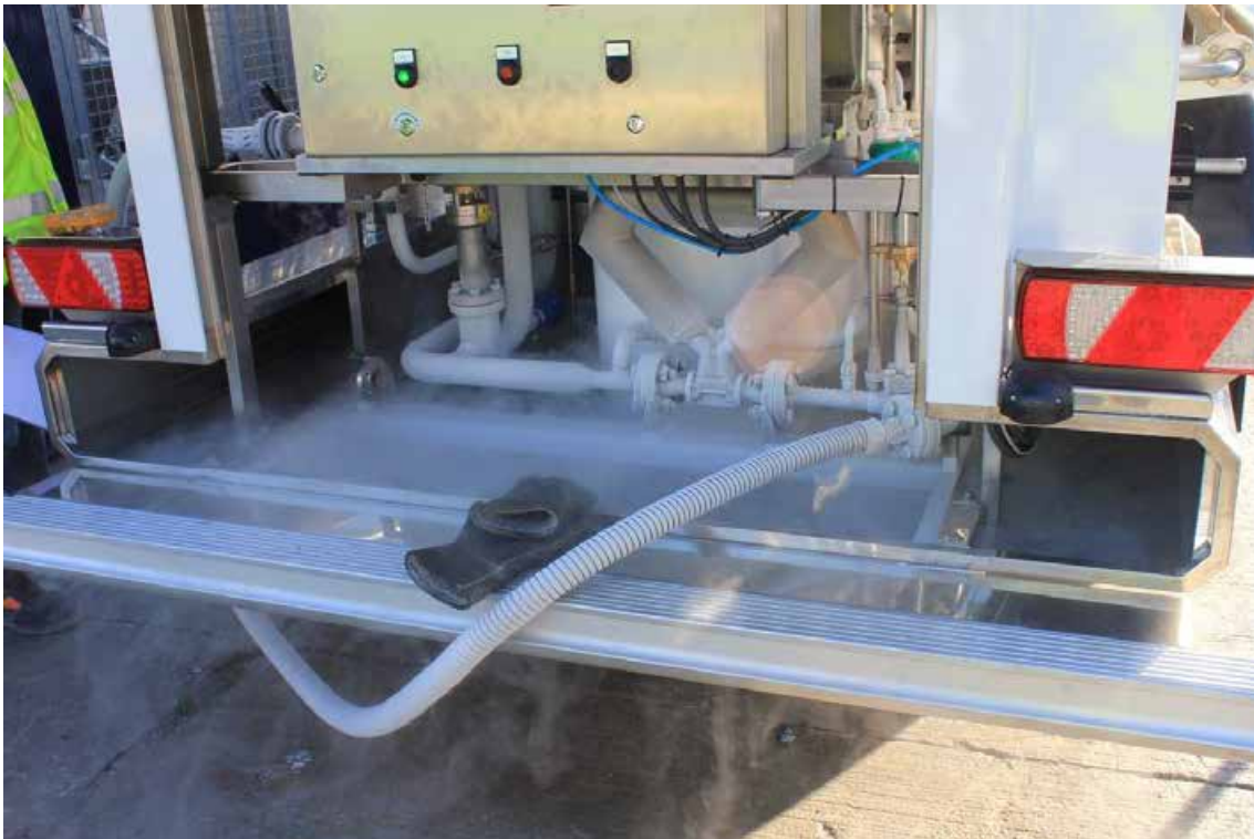
Figura 123. Tank control system. Pipes cooled by the passage of LNG to - 145°C.
