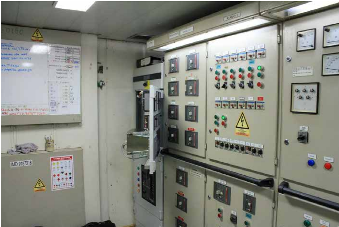
Figura 103. New ship control panel for external source of electricity.
