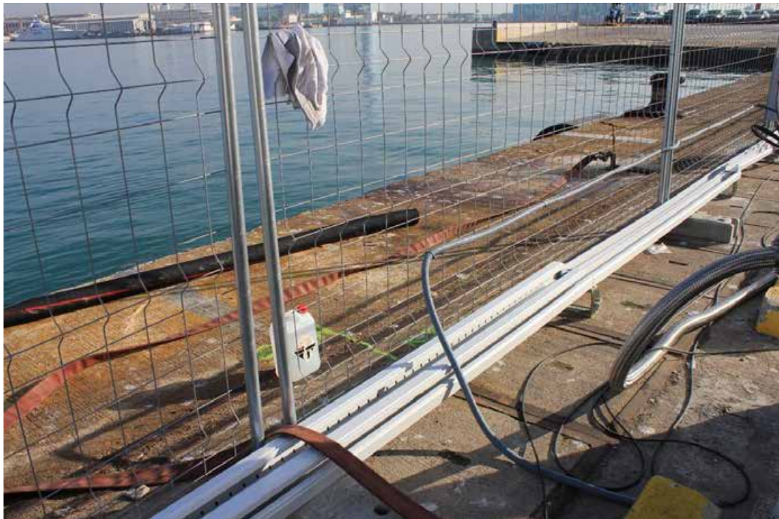
Figura 89. Surface trunking for the 15 kV wiring between the earth transformer and the connection terminal.
