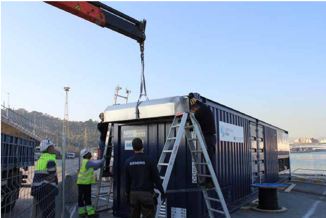
Figura 133. Installation of the ventilation air inlet module. Using the crane to hold the part in place.
