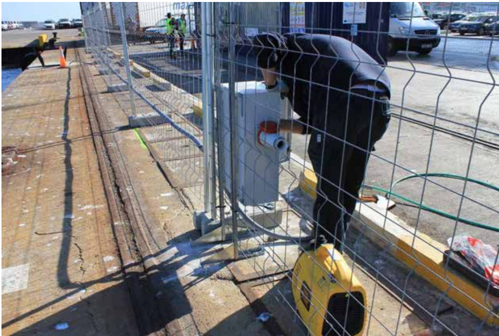
Figura 53. Installation work for the 230v connection for the tank container. Connection box.
