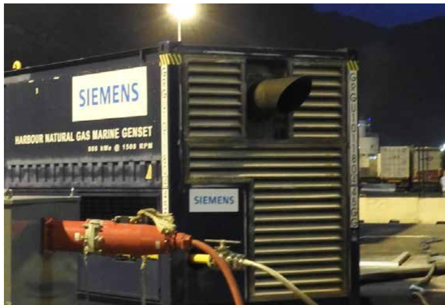
Figure 55. Installation of the exhaust gas system. The grids are part of the ventilation system of the engine room.
