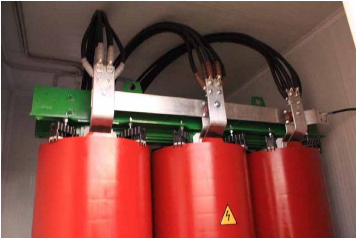
Figura 87. Earth transformer. Detail of the dry type three-phase power transformer encapsulated in resin.
