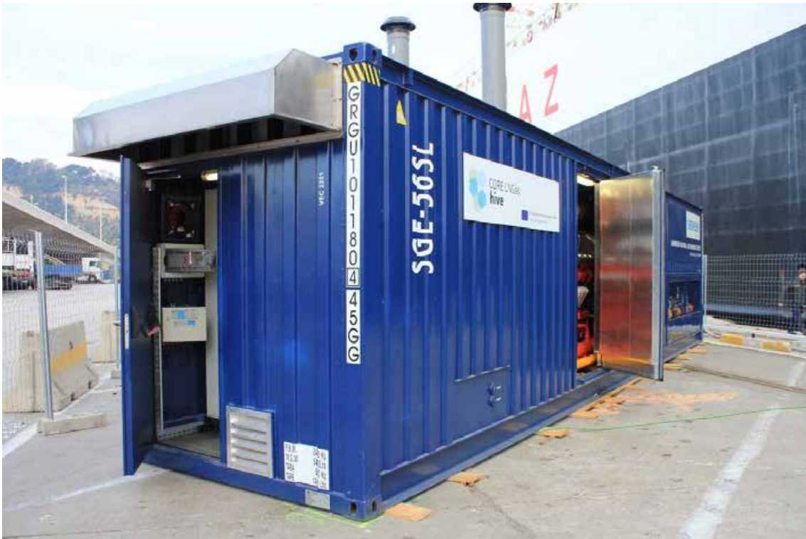
Figura 164. Pilot of 8 December. Generator engine.
