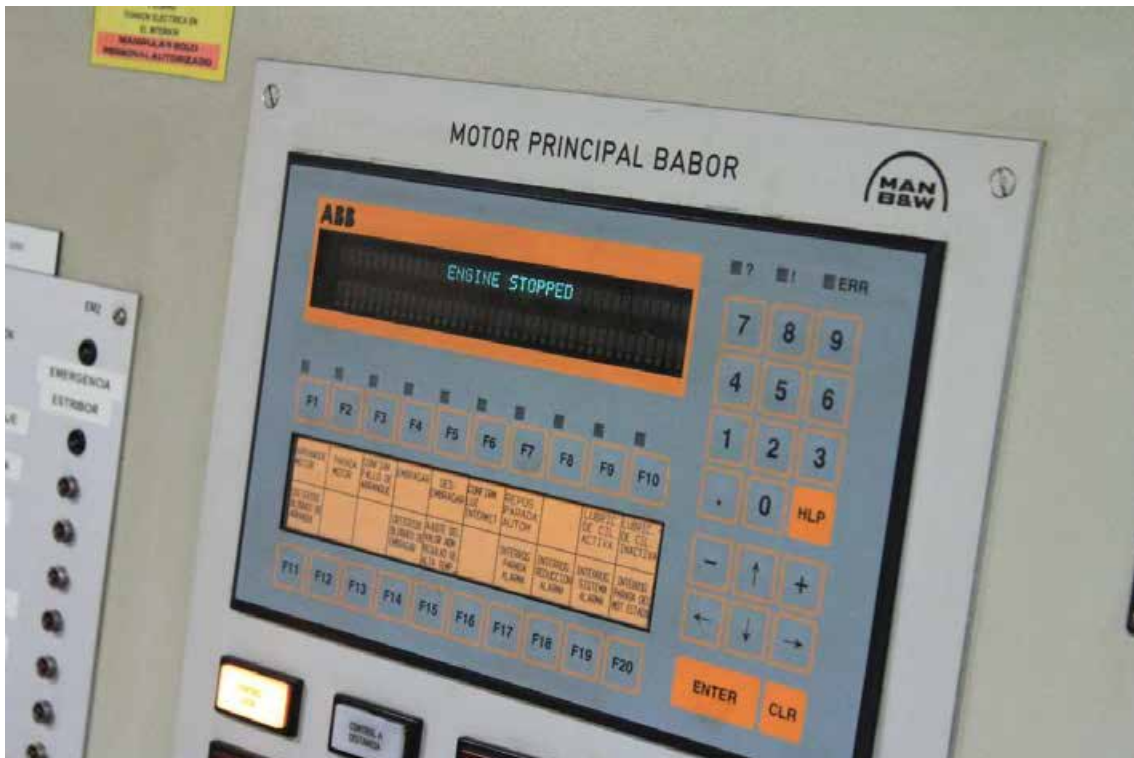
Figura 170. Pilot of 8 December. Port main diesel engine stopped.
