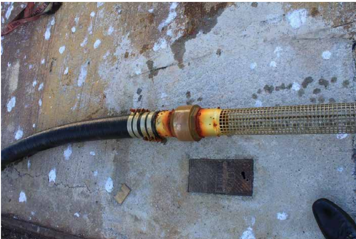
Figura 66. Check valve and filter after pilot tests. Some rusting is visible.
