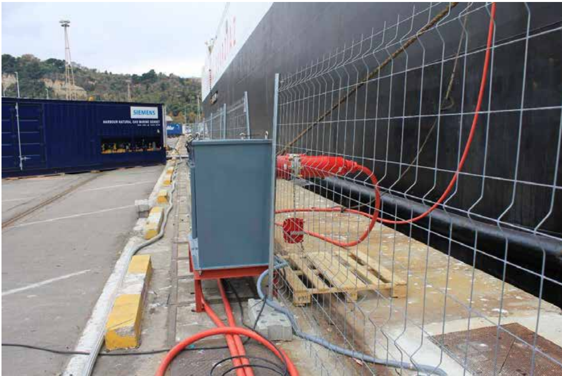
Figura 95. Connection between the connection terminal and the cable coming from the ship.
