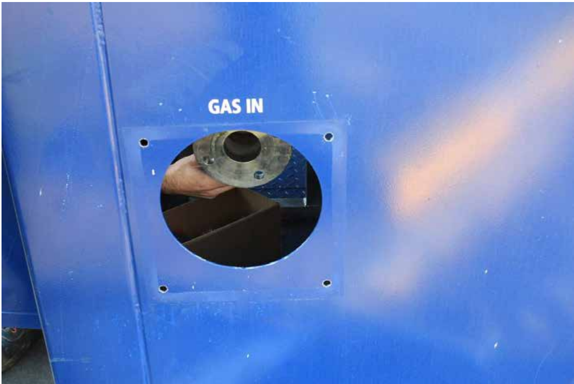
Figura 71. Gas inlet to the gas train of the engine container.
