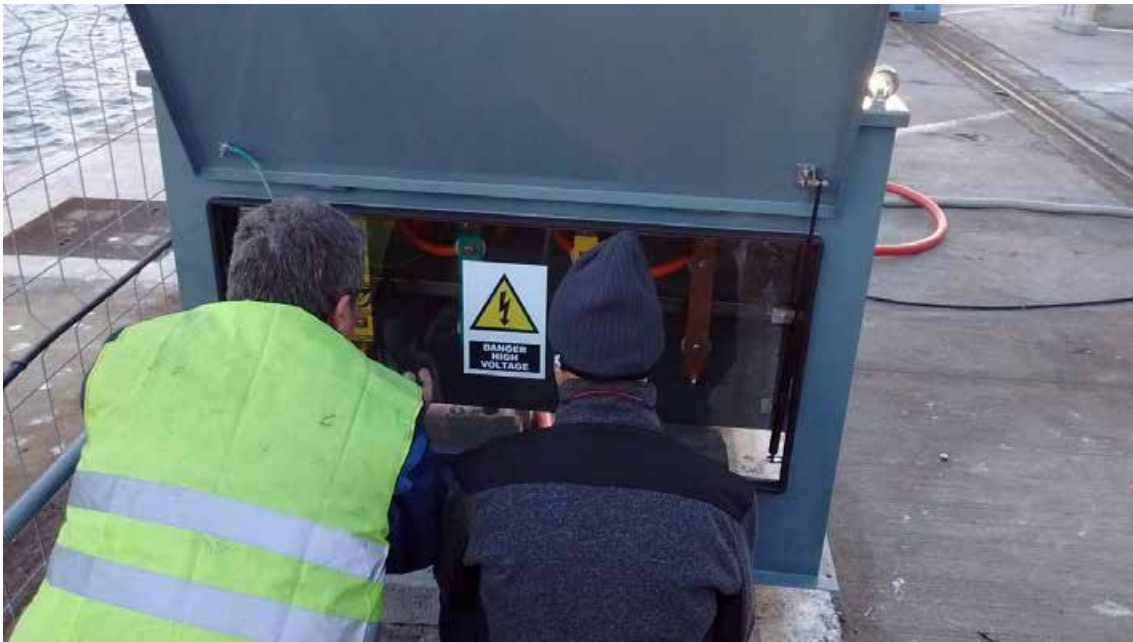
Figura 93. Connection terminal connecting bars, into which the 15 kV cable from the transformer is connected.
