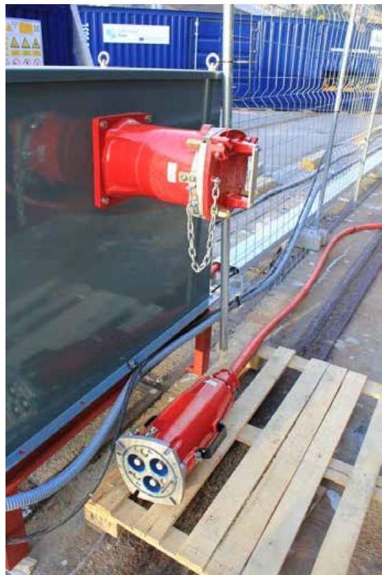
Figura 94. Detail of the connection point between the connection terminal and the cable coming from the ship.
