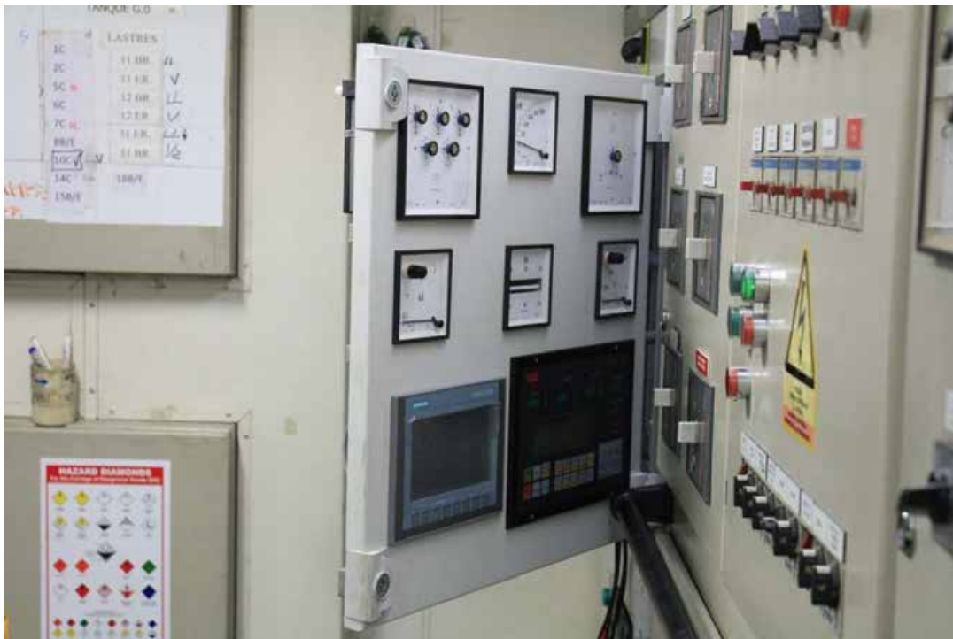
Figura 102. New ship control panel for external source of electricity.
