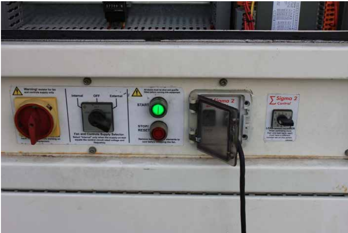
Figura 145. Resistive load bank.
