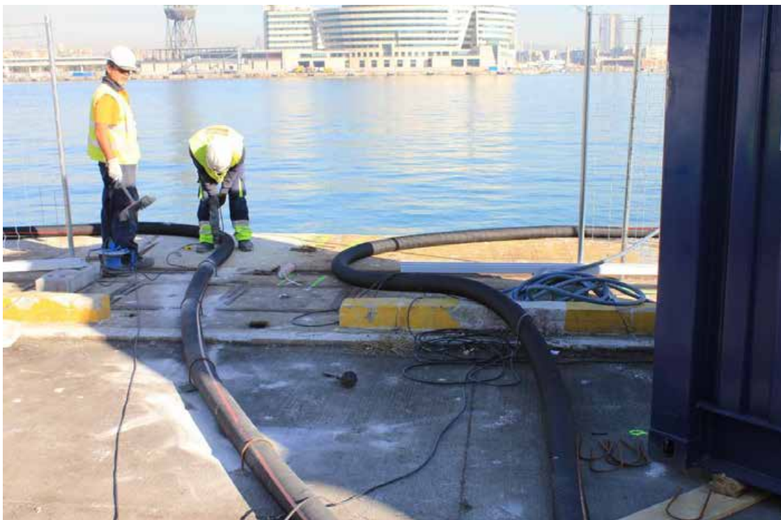
Figura 58. Installing the ND100 pipes of the secondary refrigeration circuit. Drilling holes in the concrete to insert the fixing rods.
