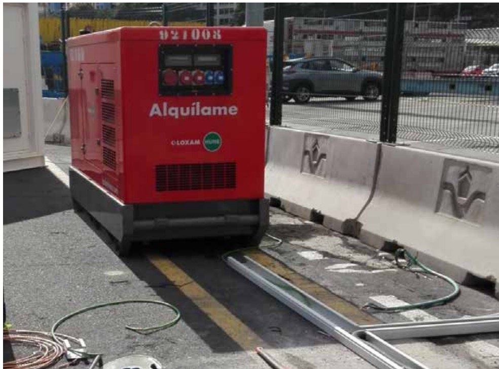
Figure 26. Installation for the 230 V connection for the tank container.
