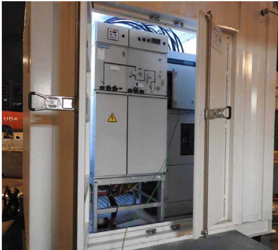
Figure 41. Transformer. Control panels.
