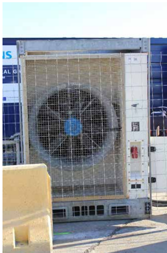
Figura 146. Resistive load bank. Fan to dissipate the heat of the element.
