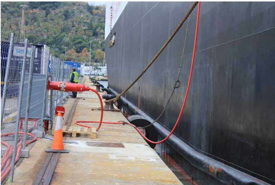
Figure 21. Electricity connection (Port of Barcelona).
