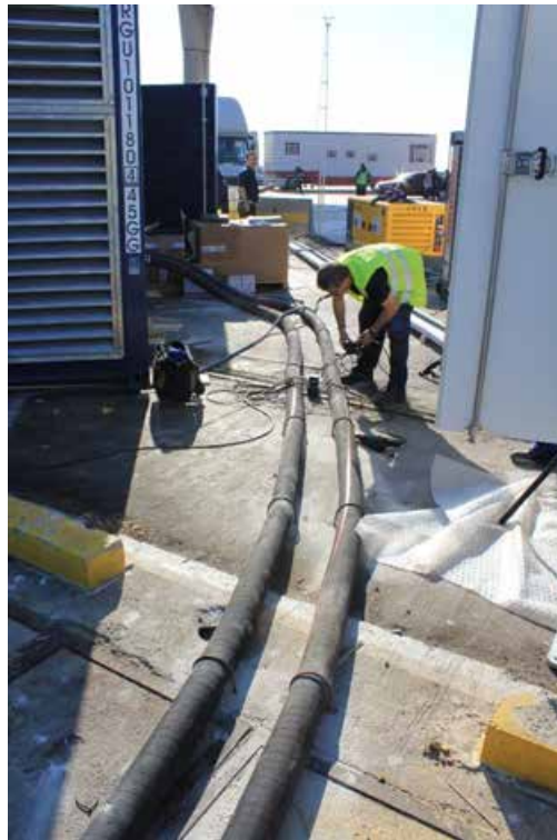
Figura 59. Installing the ND100 pipes of the secondary refrigeration circuit. Inlet and outlet pipes fixed with rods.
