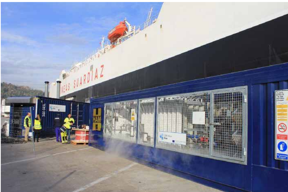
Figura 157. Pilot of 24 November. All equipment. It is possible to make out the condensation of the ambient humidity due to the cold of the LNG plant.
