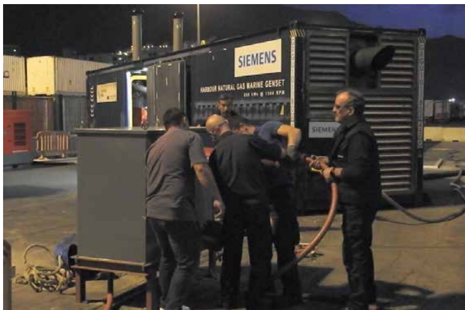
Figure 62. Pilot of the 11th of November. Connection of the medium voltage cable to Monaguillo .
