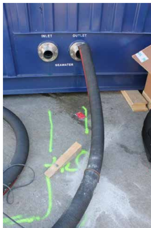
Figura 62. Installing the ND100 pipes of the secondary refrigeration circuit. Connection to container entry and exit point using flanges.
