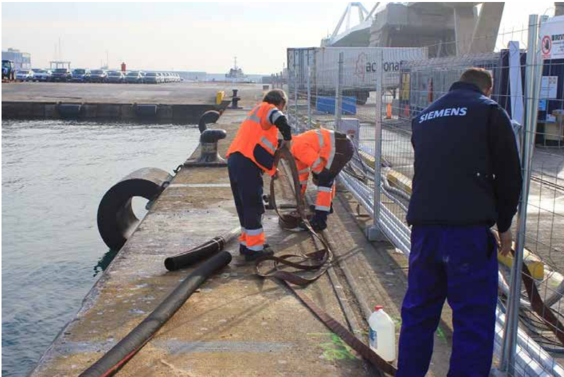
Figura 67. Operatives of the APPB Water Brigade installing a water point to prime the secondary circuit.
