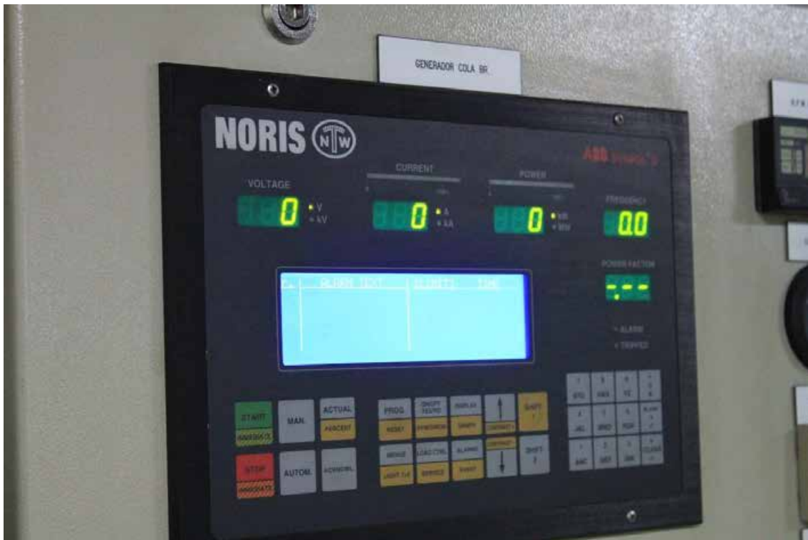
Figura 168. Pilot of 8 December. Tail diesel auxiliary generator stopped.
