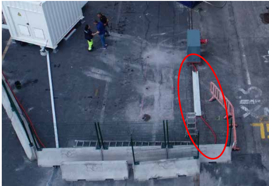
Figure 43. Superficial channelling for the 15 kV cable between the earth transformer and Monaguillo .
